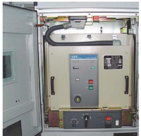
■ 断路器室 Circuit breaker compartment
